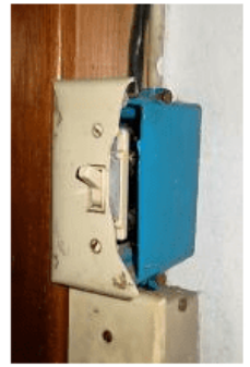
Switch cover damaged.
