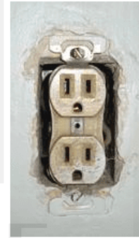
Outlet cover missing.
